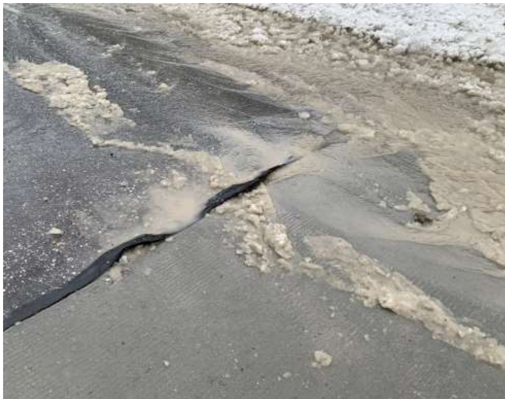
Figure 2: Bridge joint seal damage – February 2024
