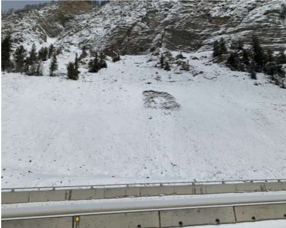
Figure 1: Slump developing on Pronghorn Upslope – February 2024
