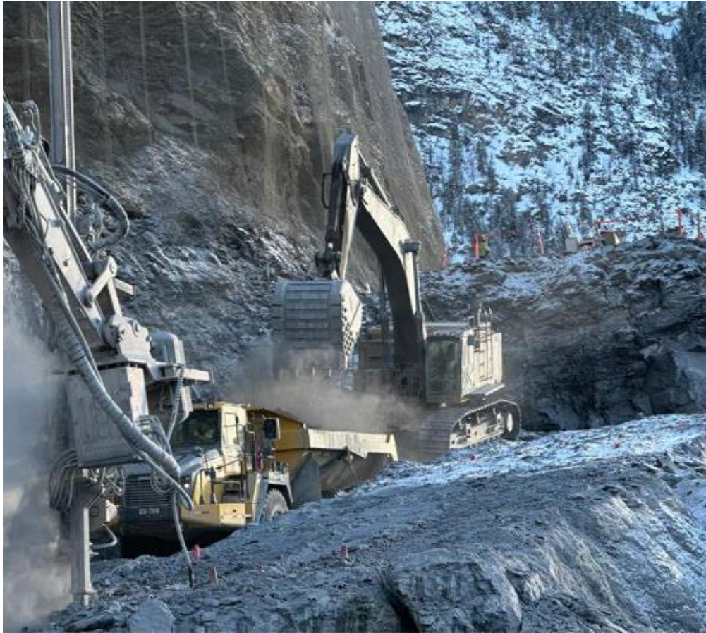
Figure 3: Cut 4 – Crews continue to load and haul blast material to disposal site – February 28, 2023
