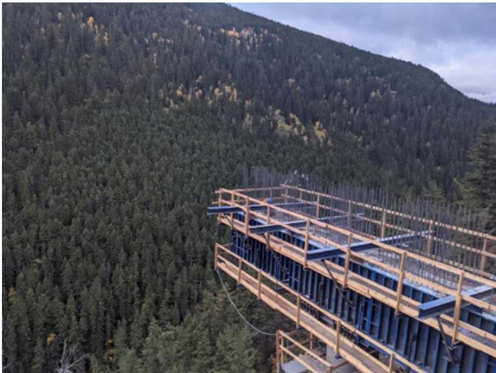
FIGURE 6: SHEEP'S BRIDGE – KHCC CREW STARTING TO REMOVE DOKA FORMS FROM PIER CAP – SEPT 30, 2021
