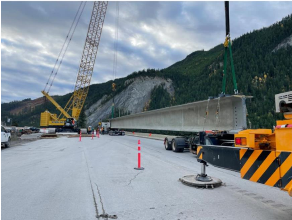
FIGURE 5: SHEEP BRIDGE, UNLOADING NEW GIRDER; LOOKING EAST FROM WEST LIMIT OF PROJECT SEPT 29, 2021
