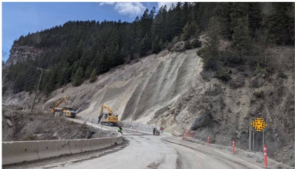
Figure 2 – KHCC crews saw cutting asphalt, hammering, and loading onto rock truck for removal at Marmot
