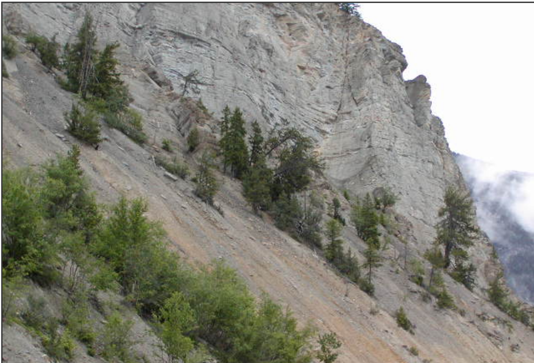
Figure 8. Consolidated bedrock and talus slope (Phase III West) above the Trans-Canada Highway.
